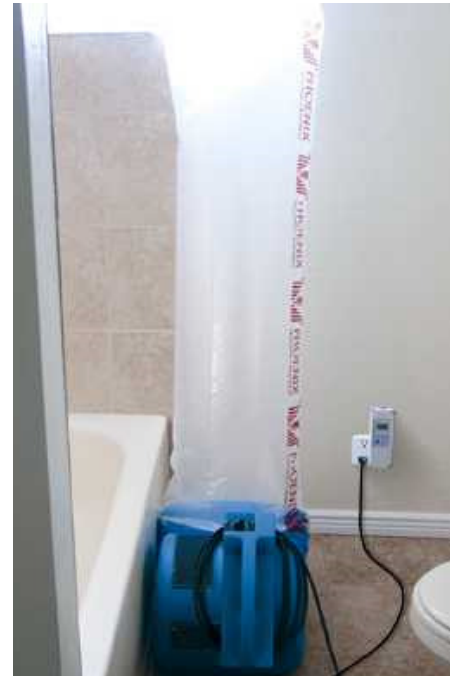
Air mover with ducting connected to Exhaust Controller
